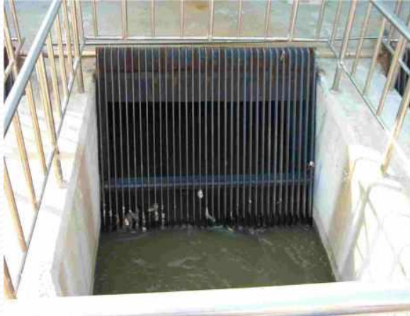
Manual Bar Screens
